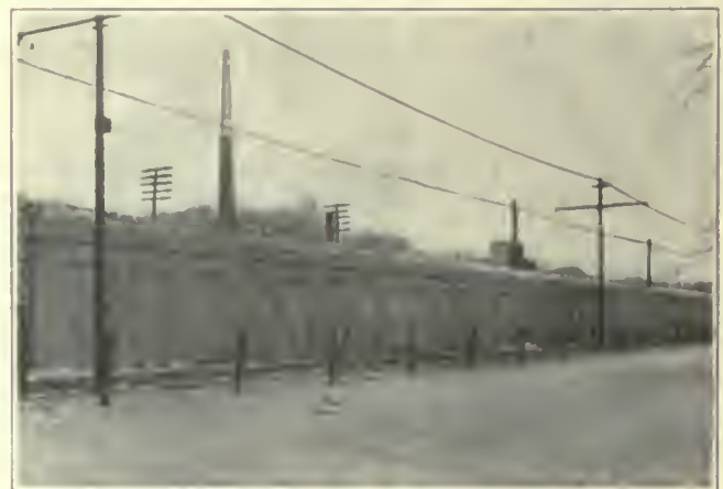
FIG. 280. TRACK ELEVATION. Concrete retaining wall of the Chicago & North Western Railway at East Avenue, Oak Park.
